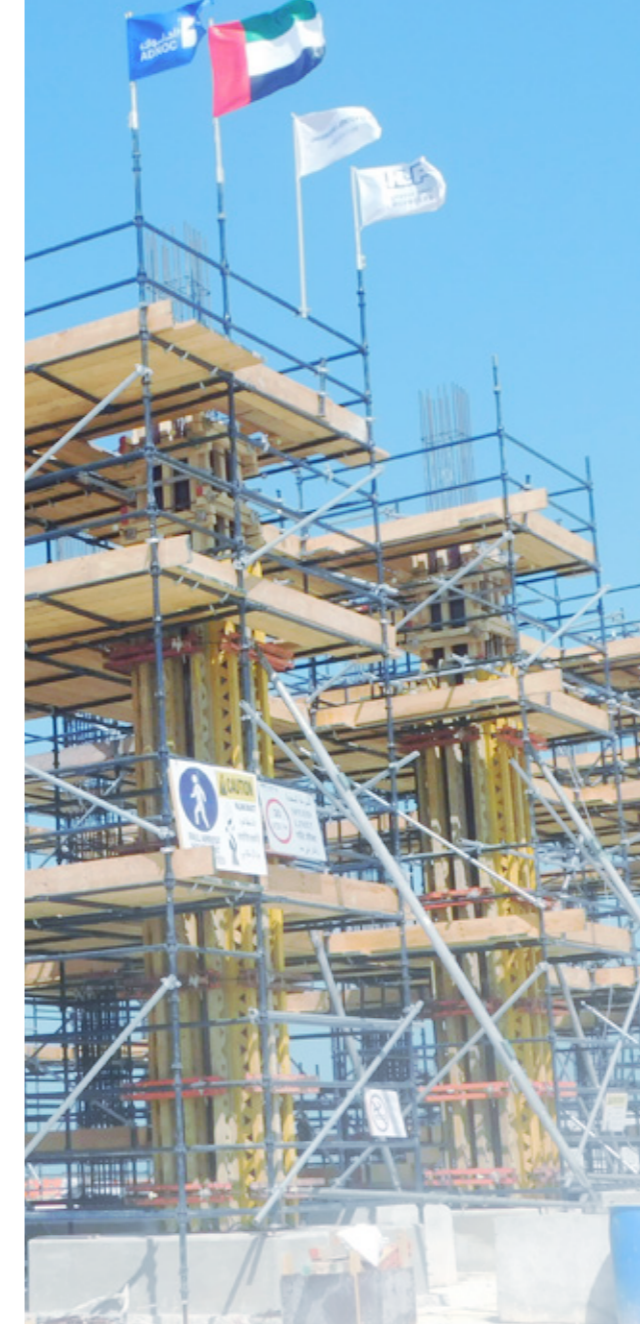
Mirfa Seawater and Supply Company
