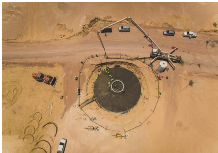
Foundation concrete works at the 250 MW wind farm in Ras Ghareb, Egypt
